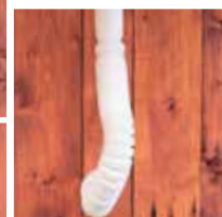
Drain sink siphon
